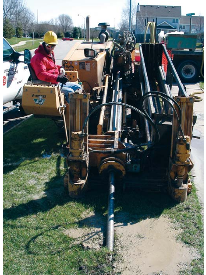
Wells Fargo commissioned Baker Electric to install two four-mile stretches of fiber-optic lines from its current home mortgage office to a planned 176-acre office campus.
